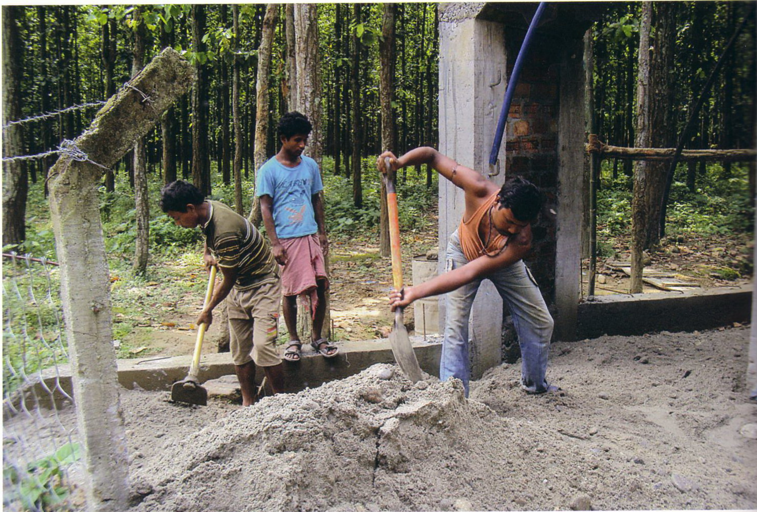
Construction is underway on a new turtle conservation center in Nepal. PHOTO CREDIT: ARCO NEPAL
